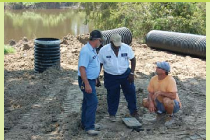
Mayor Mike Chauffe, Maintenance Supervisor Phillip Favoroth and Jim Garrett of Pointe Coupee Contractors look over work dirt work after a hazardous ditch was closed.
