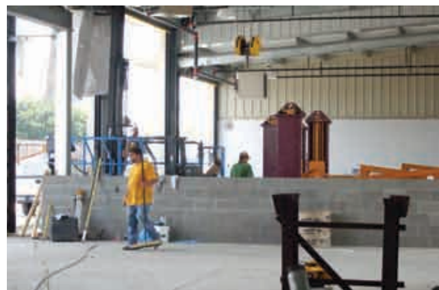
The maintenance facility project includes new concrete and the consolidation of two buildings in the rear of the complex to one facility.
