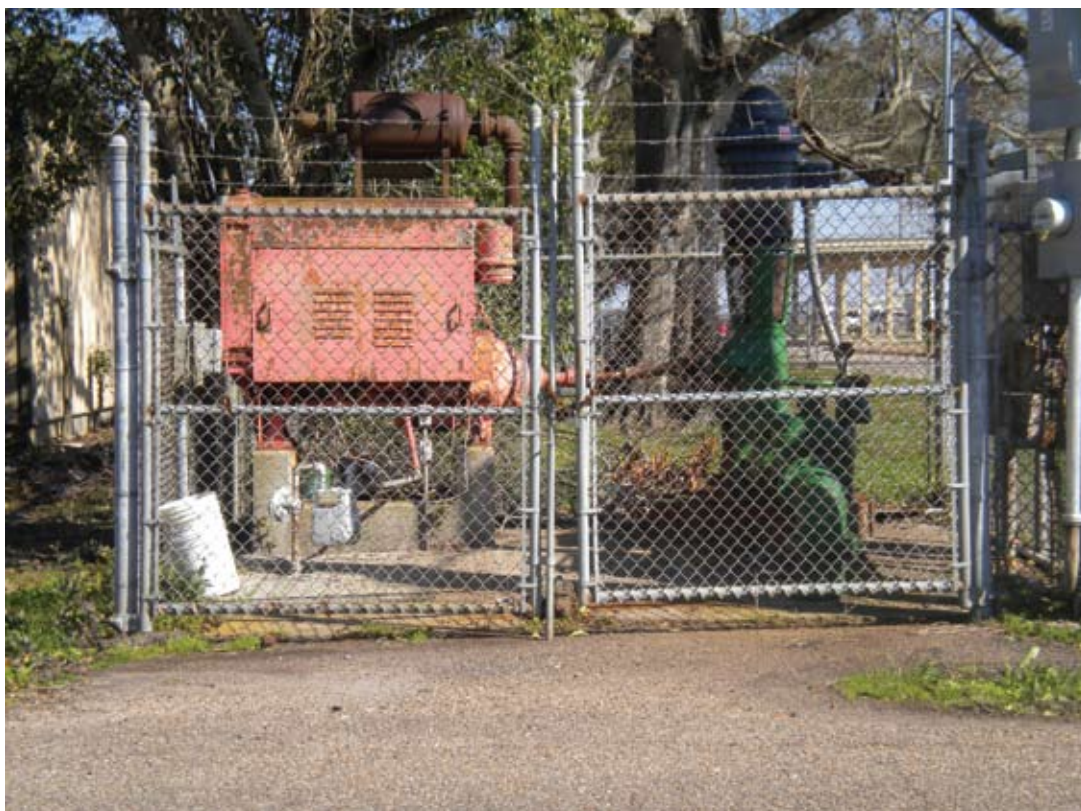
The Town of White Castle has been awarded a water enhancement grant by the Office of Gov. Bobby Jindal. The grant will cover the cost of replacing the old existing back up power supply for the water well number two, shown behind the fence in the photo above.
