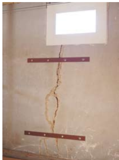
Cracks such as the one shown above were common throughout the building before its restoration.
